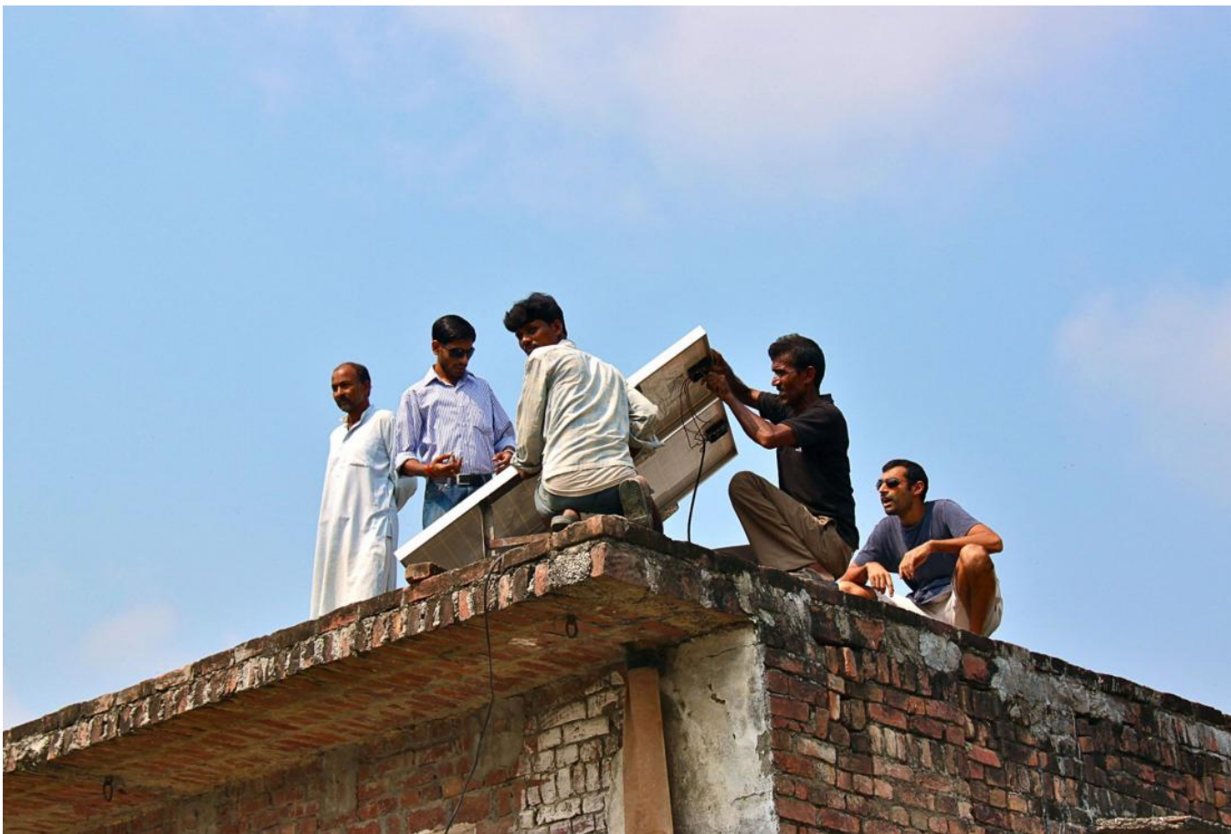
Installing a solar microgrid in India. Photo: Anna da Costa | CC BY-NC-ND 2.0
