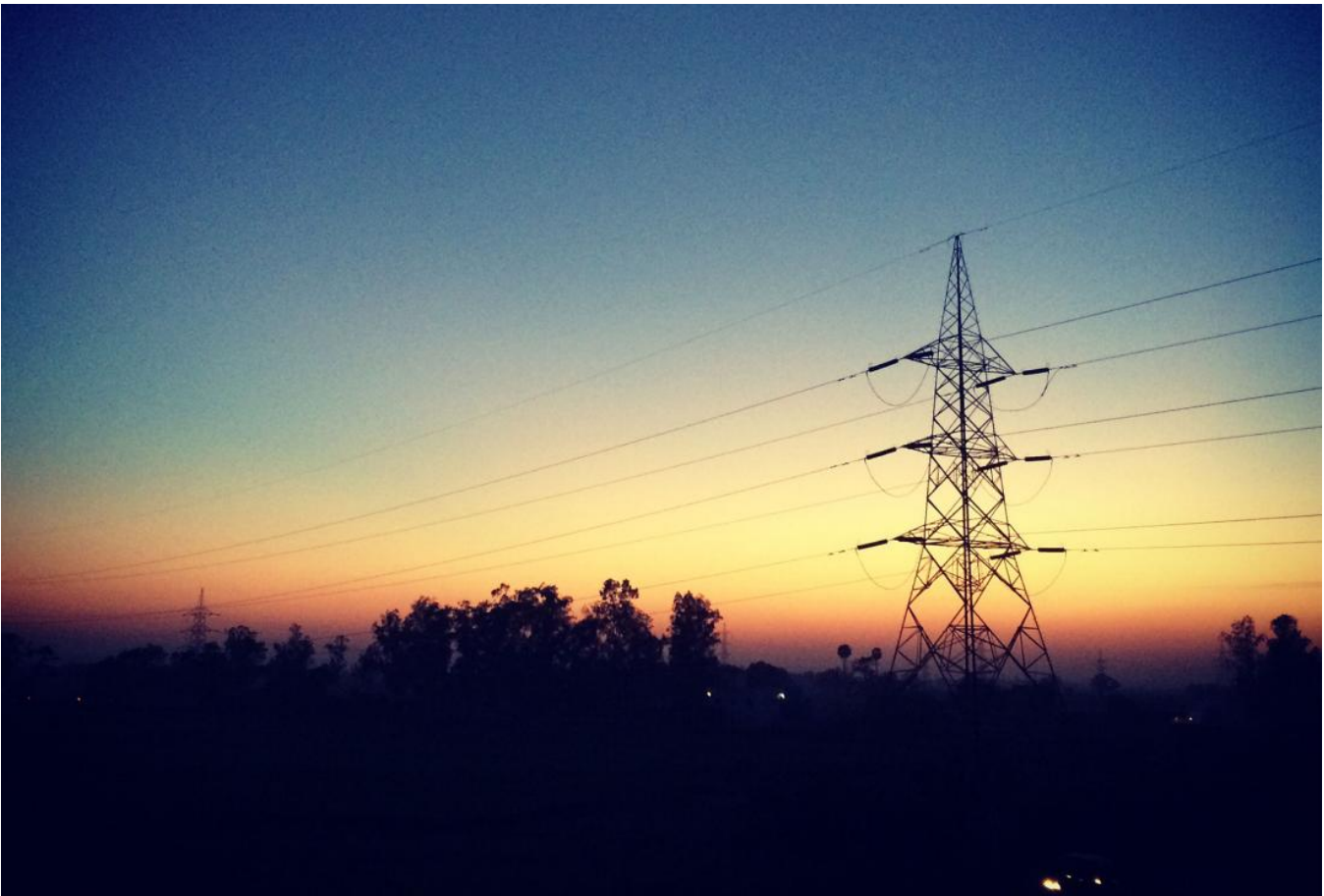
A power tower supports electrical lines in Bihar, India. Photo: Prianthi Roy | J-PAL
