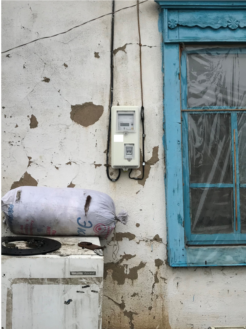
Figure A4: Example Showing Smart Meters Installed on Outside of House
